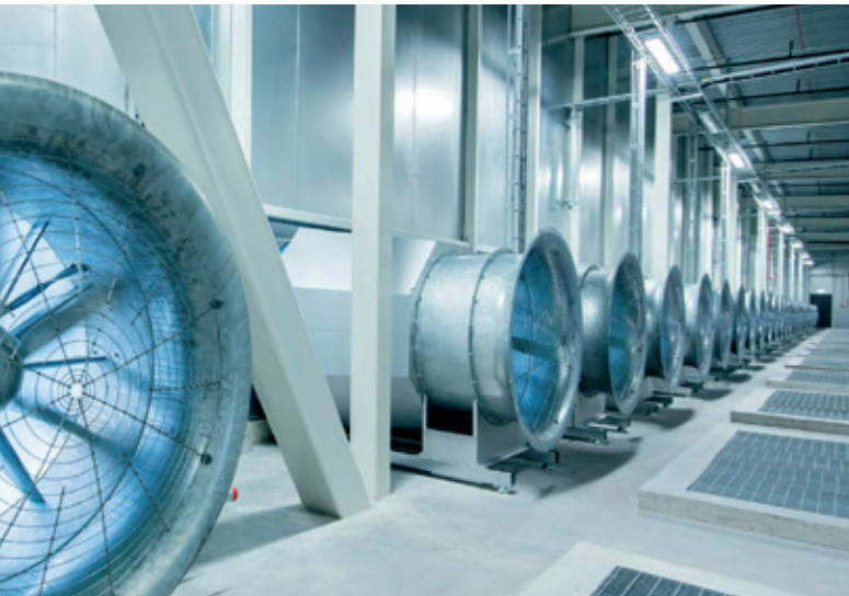
Data centre cooling system
