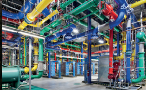
Inside data centre
